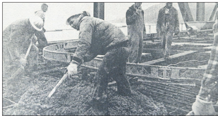
Laying of concrete deck on north spans of the Astoria bridge continued this week.
