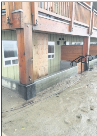
R.J. Marx/The Daily Astorian Damage from water and debris at a beachfront room at the Surfsand in Cannon Beach.
