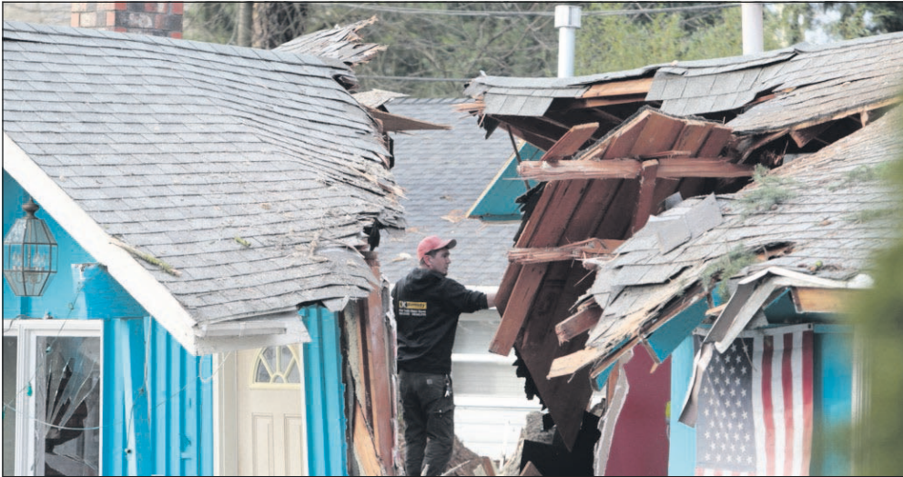
A worker assesses damage from a large fir tree that fell on a house overnight and killed an elderly woman in Portland, Wednesday.
