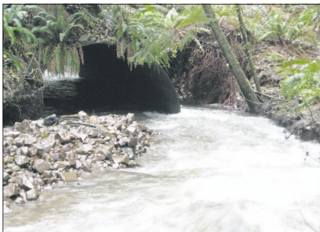
Oregon Parks and Recreation Department Canyon Creek rushes through a culvert under Ecola State Park Road. Heavy rainfall eroded the earth under the road near the culvert, prompting park officials to close Indian Beach.
