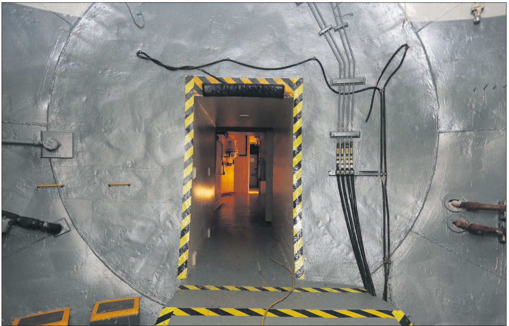
A tunnel leads to an underground bunker housing the launch control center at the Air Force’s Quebec-01 Missile Alert Facility north of Cheyenne, Wyo. The Air Force has been restoring the missile alert facility as a state historic site.
