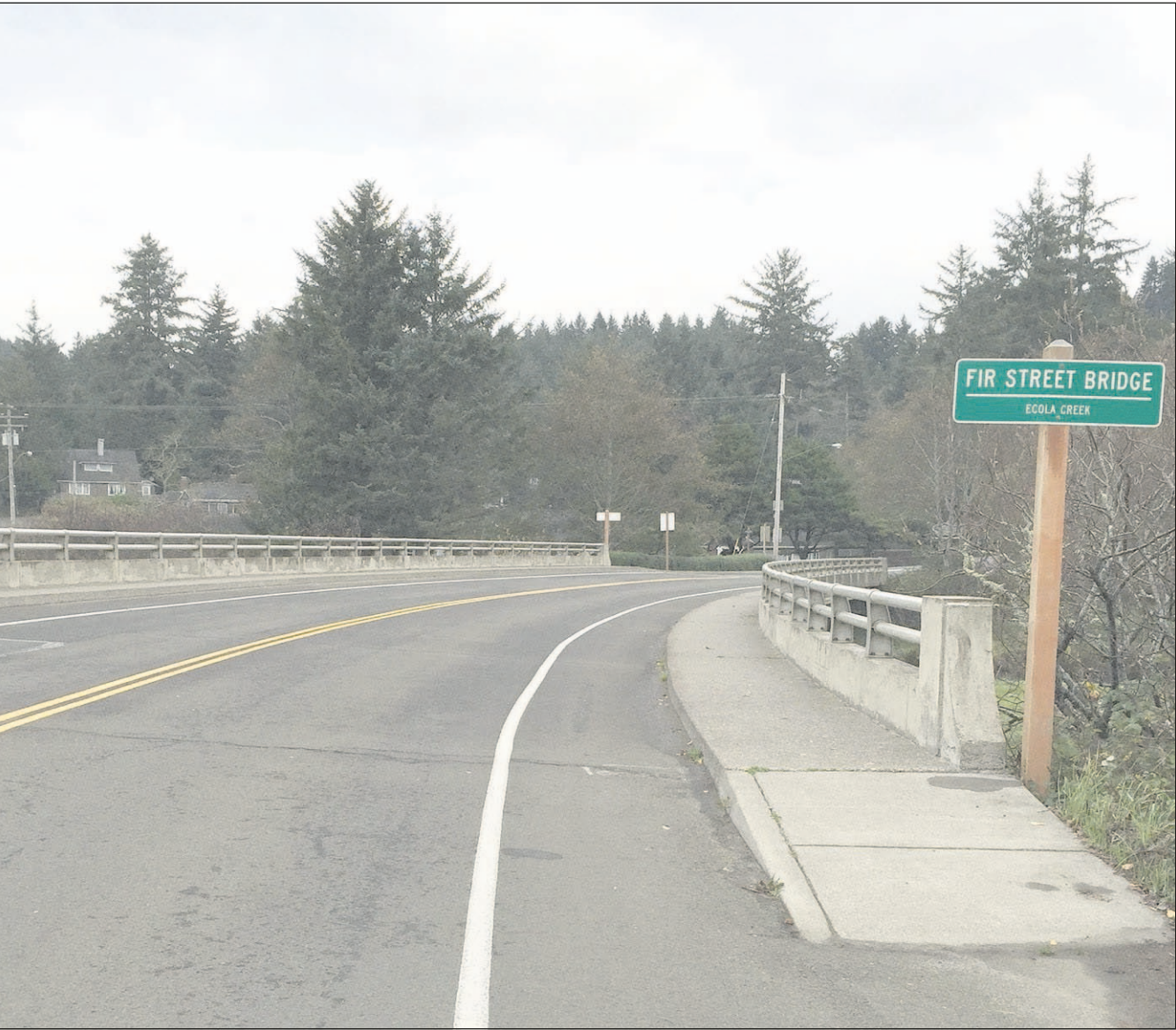
The Fir Street Bridge is expected to fail during an earthquake or tsunami.
