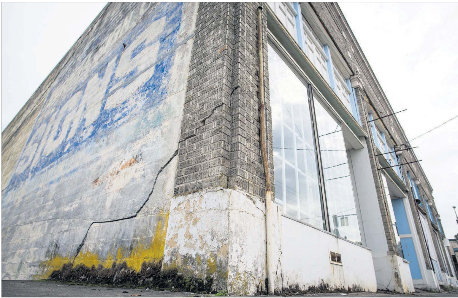
A crack in the M&N Building is visible from Ninth Street.
