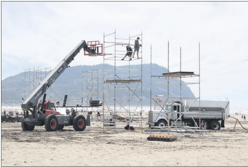
Crews were busy Tuesday afternoon setting up the beach, just north of the Seaside Turnaround, for the Hood to Coast and Portland to Coast Relays’ “finish party” Saturday. Runners will flow in throughout the day and be treated to live music, food, drinks, vendors and a party-like atmosphere.
