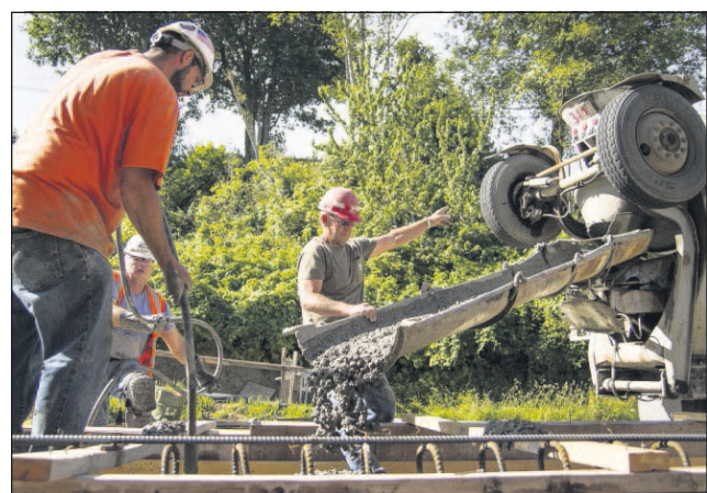
JOSHUA BESSEX — The Daily Astorian From left, Dave Embree, Rodney Wendel, and Frank Berg, pour concrete on the Irving Avenue Bridge Tuesday. The $5.8 million replacement of the bridge is 90 percent federally funded with the last 10 percent paid for by the city.
