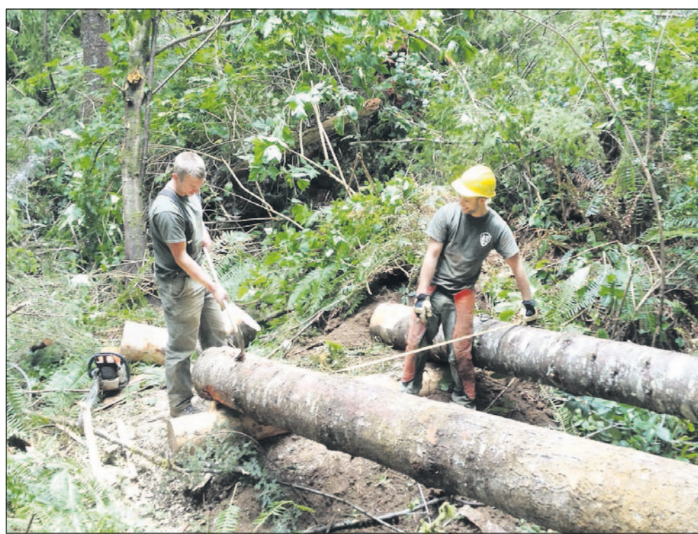
In this 2013 photo, Doug Graham, left, and Josh Fry, right, construct boardwalks to go over creeks and marshy areas along the Kwis Kwis Trail.
