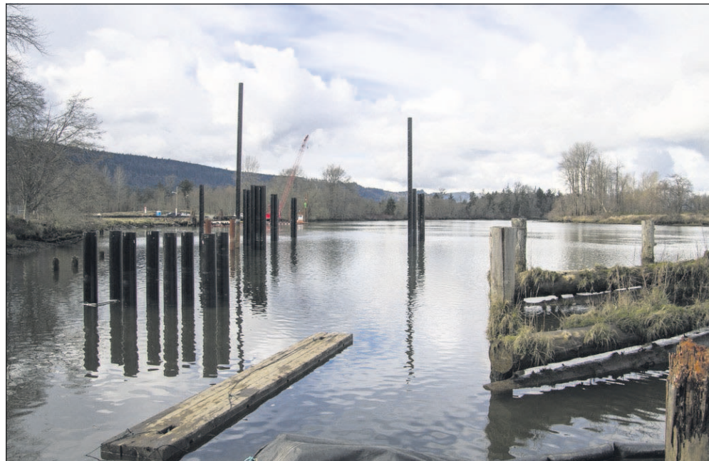
JOSHUA BESSEX — The Daily Astorian The new Westport Ferry Landing is expected to be completed by May 1 of this year.
