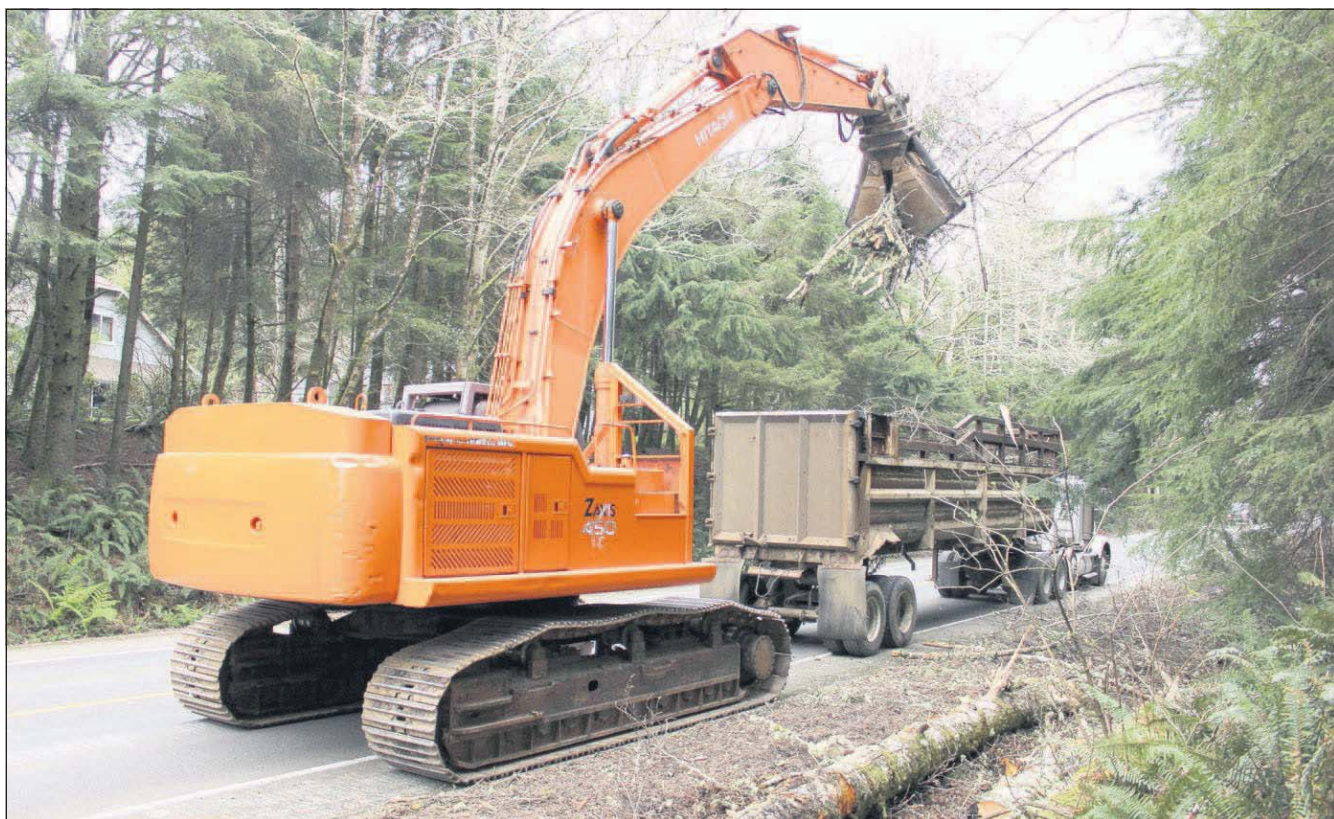
An excavator prepares to drop felled trees and brush from the east side of U.S. Highway 101 into the back of a truck. The equipment belongs to Trails End Recovery, a Warrenton-based company.
