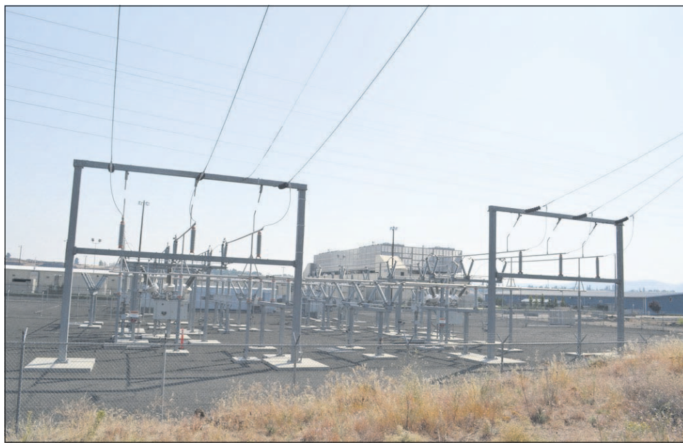
The Google data center in The Dalles.
