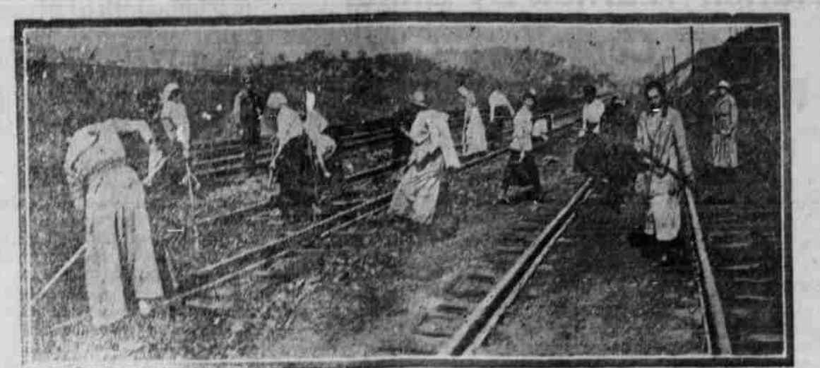
This photograph was taken on the Pittsburgh division of the Pennsylvania railroad east of Sumnerhill. Women, it proves, have actually taken up the hard work heretofore performed by men. They clean the tracks of the road, and it has been said by officials that they keep the tracks cleaner than did the men they supplanted.
