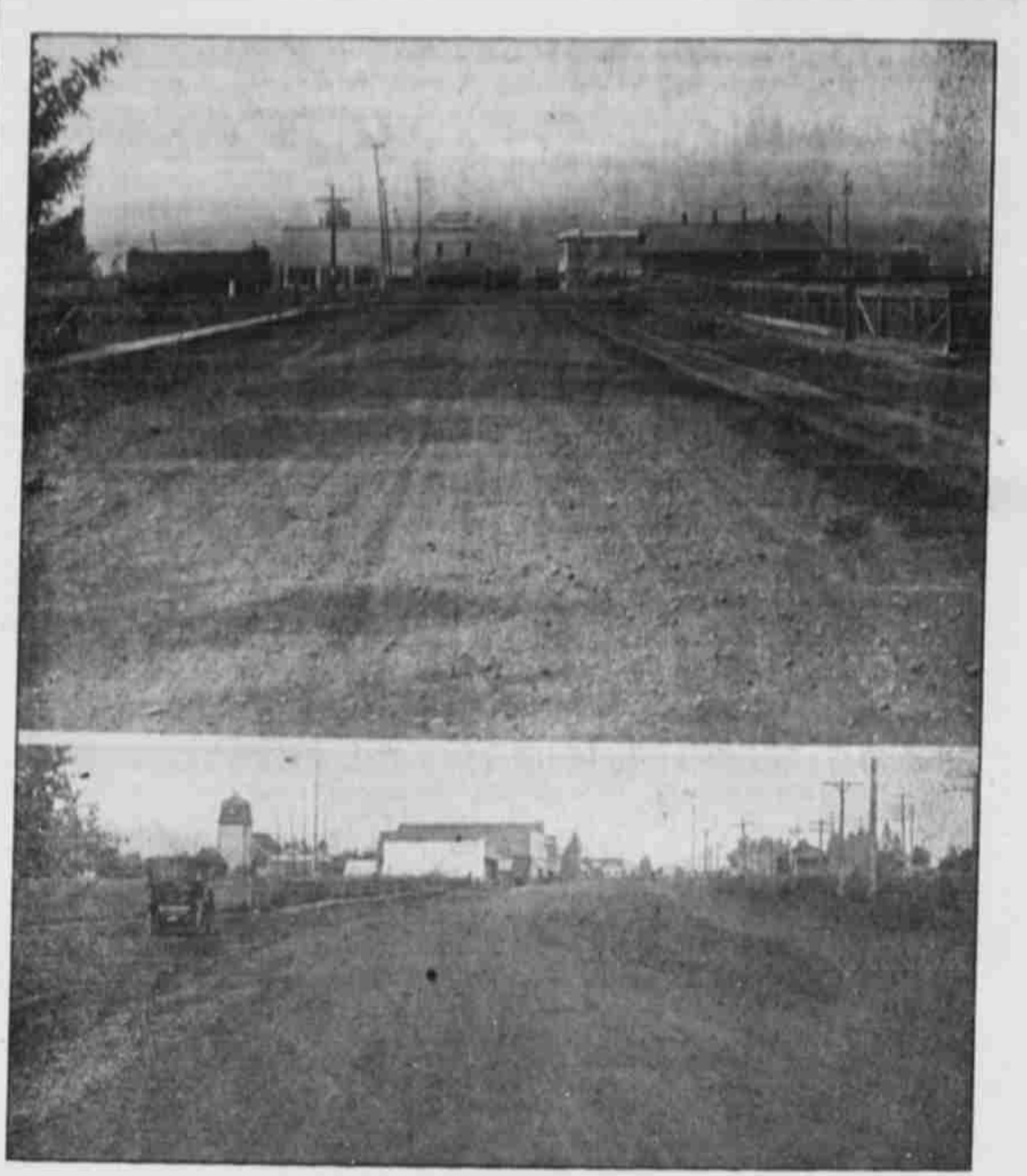
Upper picture shows street in Scappoose, Ore., which was not improved with Richmondite, and lower picture a neighboring street surfaced with this material. The street improved with Richmondite was in the same condition as the street in the upper picture.
