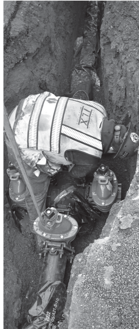
Keizer public works employee Alex Stoddard checks the new water line fittings. Photo by CHARLES GLENN of Keizertimes
