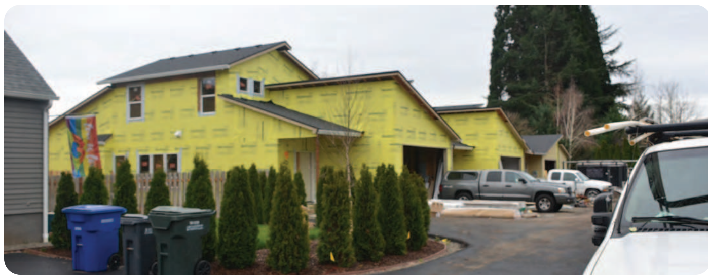
Keizer residents may soon see more multifamily housing construction projects like this one on on Sunset Ave. North. City officials say this project was already planned and is not part of the HB 2001 zoning changes. Photo by CHARLES GLENN of Keizertimes
