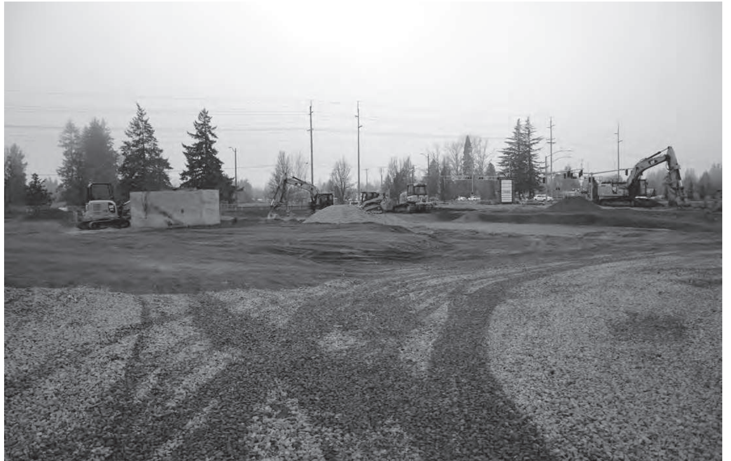
Crews from Rich Duncan Construction are in the infancy stages of building the Willamette Valley's first Chick-fil-A.
