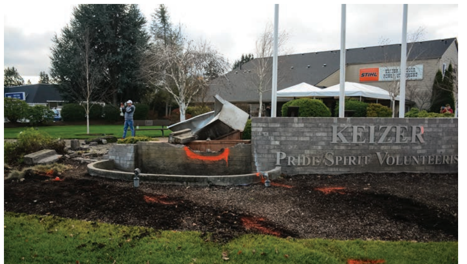
The accident damaged the brick water fountain at the corner of Chemawa and River Rd. N.
