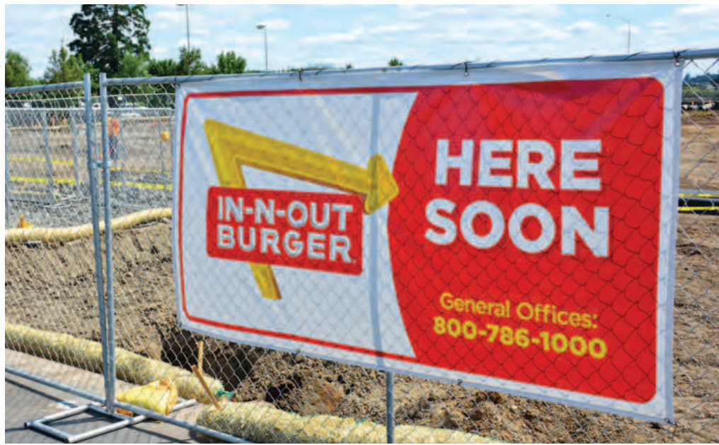
Construction of In-N-Out began in earnest earlier this month. Expect a sixth-month wait to order that double-double. KEIZERTIMES/Eric A. Howald
