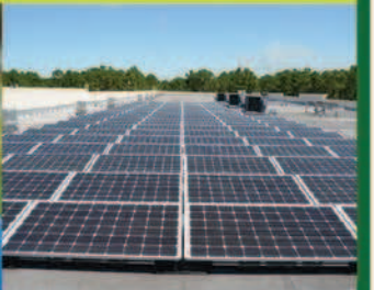
Enzymedica Solar Panels
