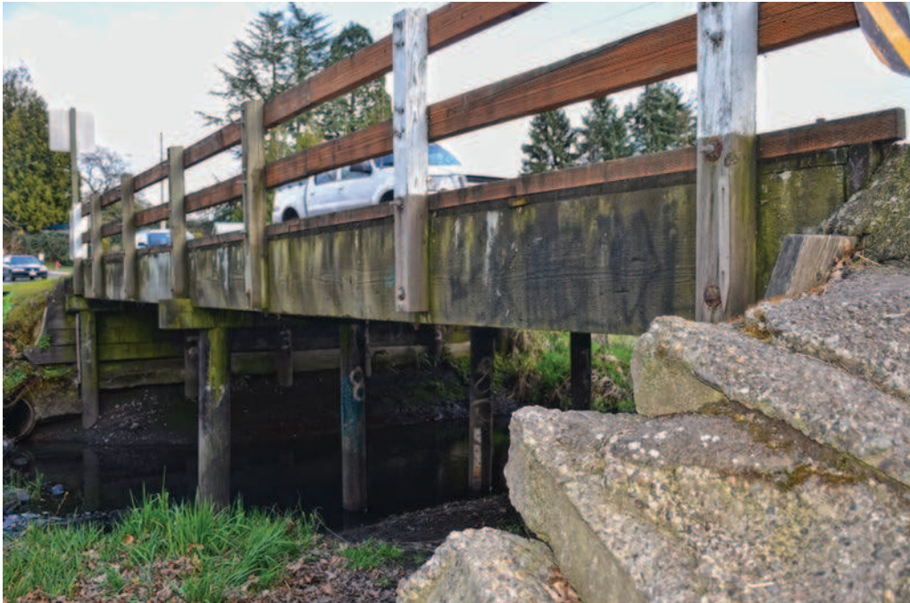
The bridge spanning Claggett Creek on Dearborn Avenue Northeast will be replaced this summer.
