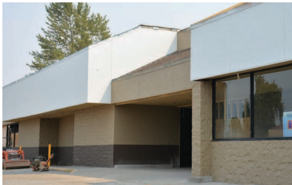
Despite a multi-million dollar remodel, Winco refused to make changes bring the parking lot up to code. A plan to leverage future developments is making its way through city processes.
