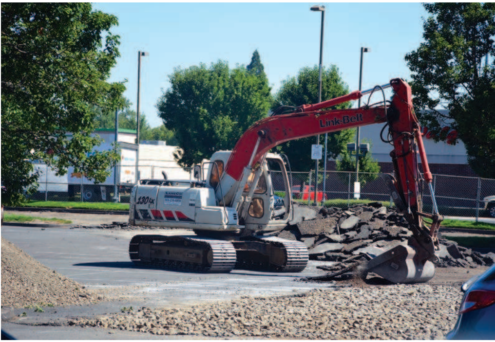
Construction crews began removing sections of the parking lot at Schoolhouse Square this week, setting the stage for a new coffee house and sandwich shop. KEIZERTIMES/Eric A. Howald
