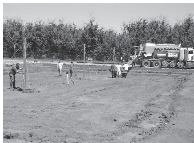
KEIZERTIMES/Craig Murphy A crew of volunteers help lay the foundation for three new sand volleyball courts at Keizer Rapids Park. Hans Schneider put the project together.
