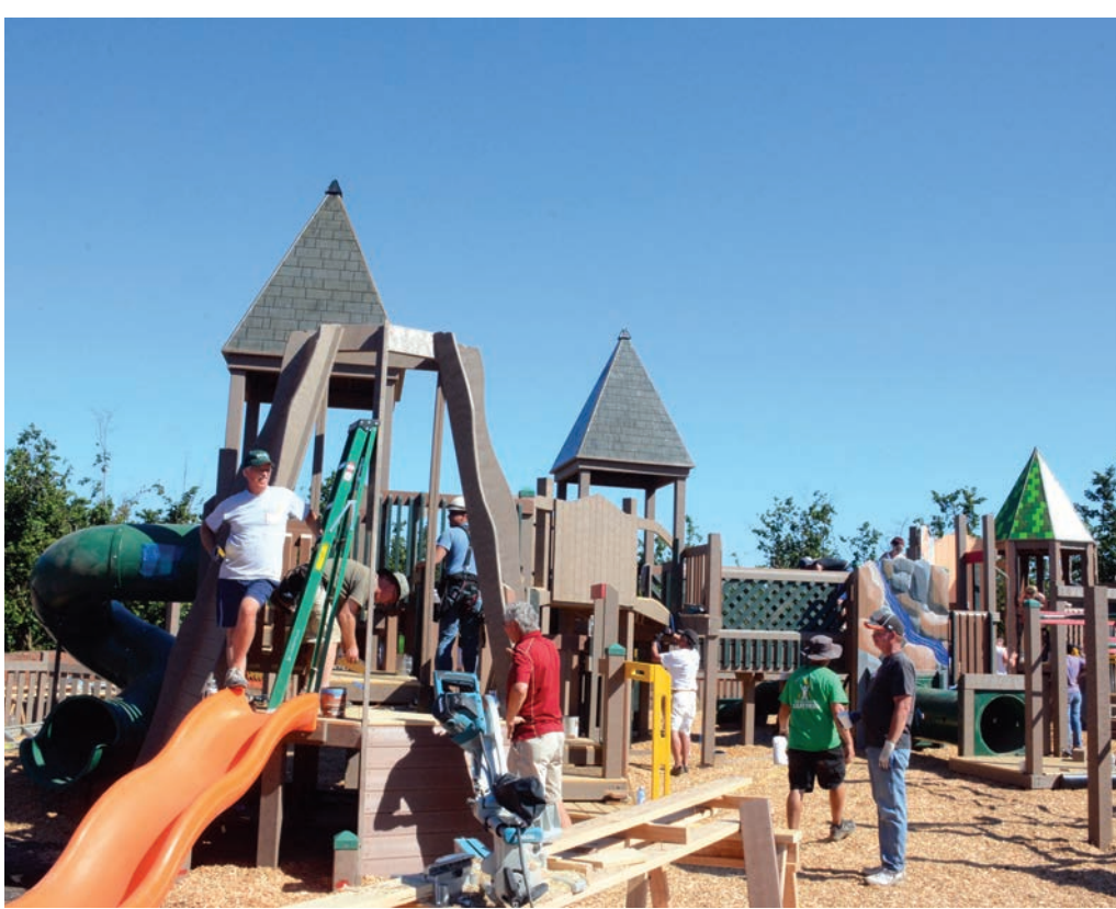
Top: Bill Lawyer and members of the Marion County Fire District No. 1 look over a tube on Friday morning that caused headaches before being trimmed to fit. Above: Volunteers work on the volcano slide and other parts of the Big Toy project on Sunday afternoon.
