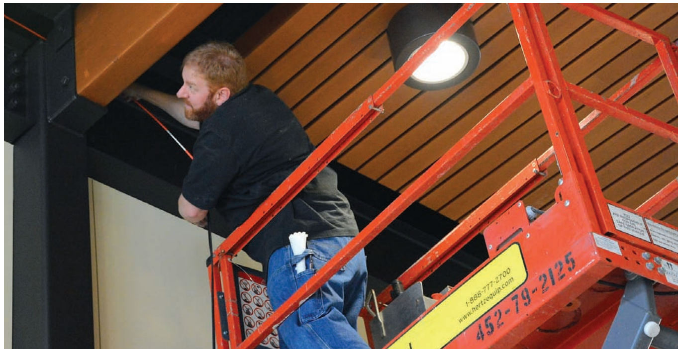
KEIZERTIMES/Craig Murphy Jason Hogan installs wiring for new cameras at Keizer Civic Center on Monday. New cameras are being put in to monitor activity in the building since the City Hall Gallery is being utilized more.
