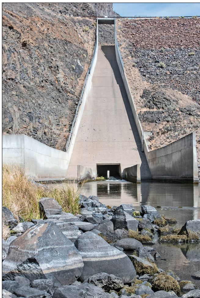
Water flows from Prineville Reservoir through Bowman Dam and into the Crooked River on Friday.
