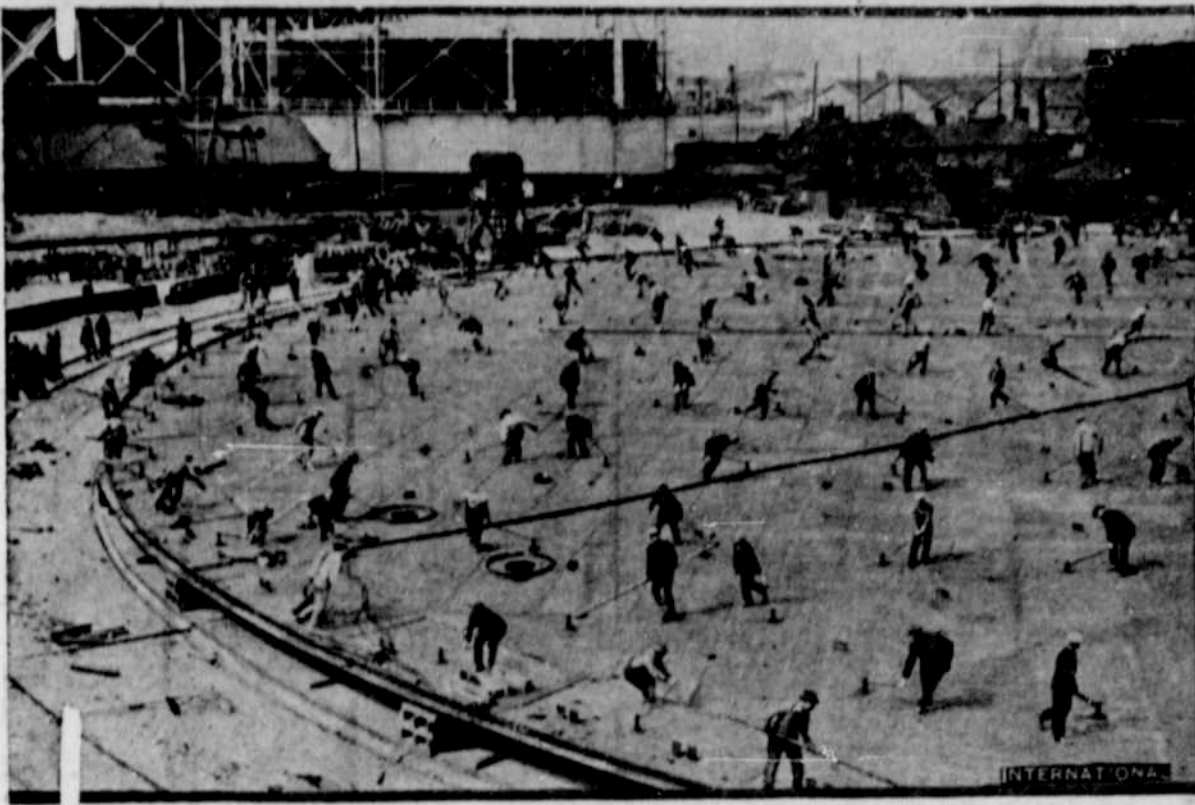
More than one hundred workmen lowering the huge base of a 10,000,000-cubic-foot gas tank for the Pacific Gas & Electric company into position in San Francisco. The tank will be 228 feet high and 276 feet in diameter. It will be of the telescopic type, having five collapsible sections.
