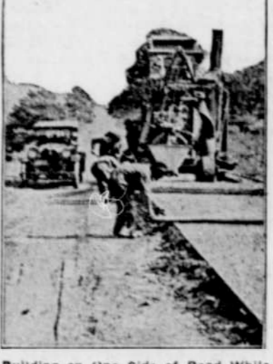
Building on One Side of Road While Other is Open to Traffic.
