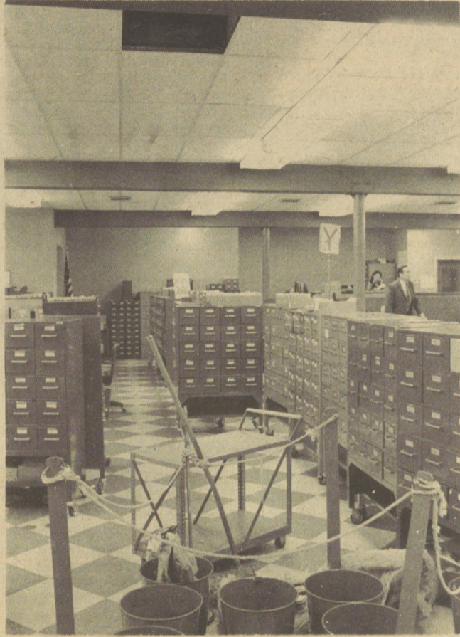
The day the roof fell in
