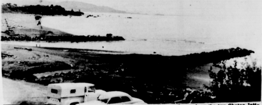
A CHANGE IN THE RIVER MOUTH is shown here pictorially, as the work on the two Chetoo Jetties progress, despite the inclement weather. Both jetties will be built out further, and built some higher. The sand bar between the two jetties may wash out this winter, the engineers feel.
