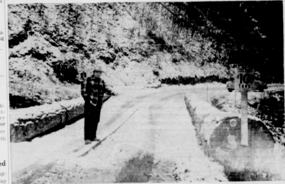
COUNTY COMMISSIONER FRED FLYNN points to sagging bridge on South Bank road across Jacks Creek. Sign report limit of 10 tons on bridge. Flynn says that the bridge will have to be rebuilt and hopes county can do it on a permanent basis. Timbers underneath have rotted away.
