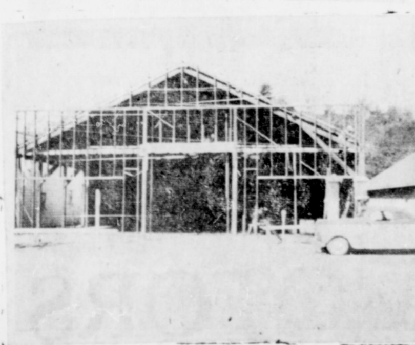
WORK IS NEARING COMPLETION on these two latest additions to making Brookings one of the most modern communities in the area. Above, Ed Lee's will move into the Morton Building next week, below, the old Azalea Garage building is shown before crews started to put the new front on the completely remodeled structure. Pilot Photo
