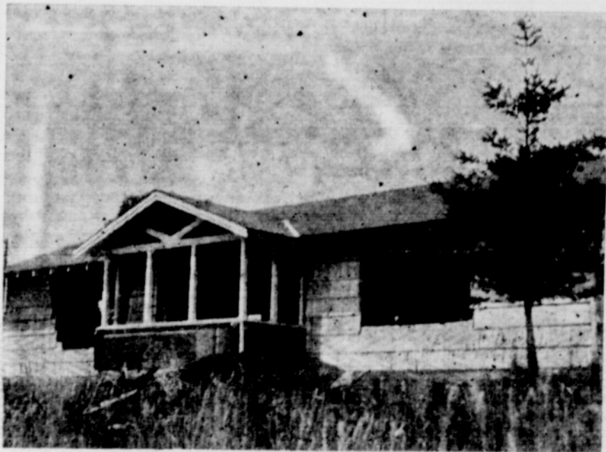
WORK IS PROGRESSING slowly on the new library building under construction in Brookings by members of the library association, and others interested in seeing that the city has a library. The land was given to the association by the Federal government, and will in turn be deeded over to the city. Almost all of the work done thus far was done on a volunteer basis by members of the association.
