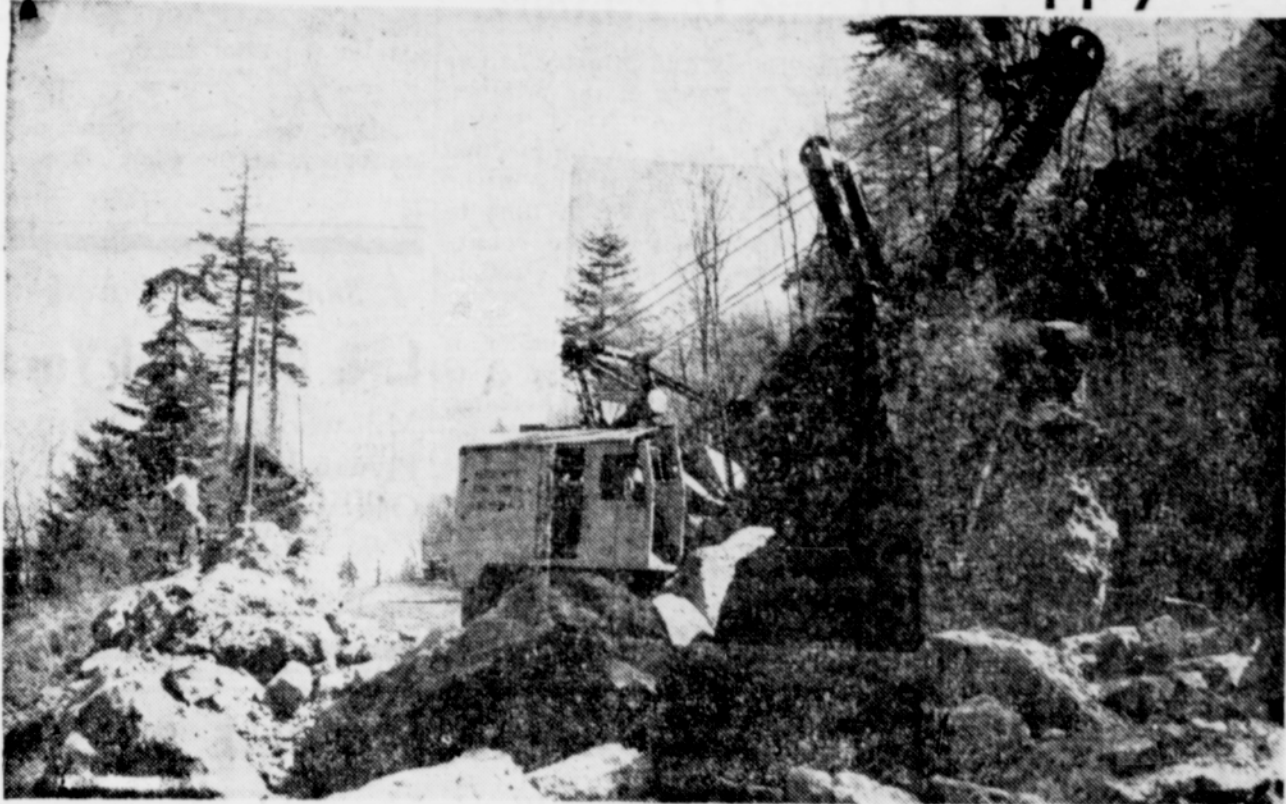
In the days of Samuel Lancaster and the other Highway Pioneers, the scenic loops and curves and grades of the Columbia Highway were built far above the river, with picks and shovels, fresnos, mules and men; also black powder, star drills and a sledge. But, when the Moderns ironed out the curves, they did it with huge suction dredges, dynamite, bulldozers and deisel oil. They made the barn-sized boulders into base material to fill the low spots until now you never feel a bump when you ride the road between Dodson and Bonneville where the boulders blocked the way when the above picture was taken. Construction like that costs approximately a third of a million dollars per mile.
