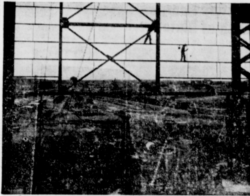
NEW STEEL FACILITIES TAKE SHAPE —Workman painting braces on the end of a new open hearth building. This new plant is part of the National Production Authority's program for the expansion of basic industry. It will play a major part in raising our steel capacity to 120 million ingot tons by the beginning of 1954.
