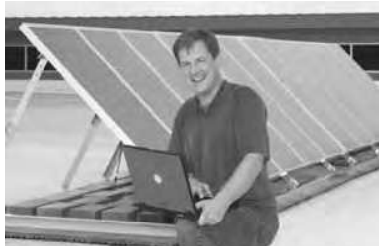
Monitoring Photovoltaic Performance at LCC
