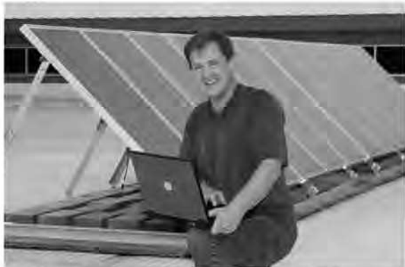
Monitoring Photovoltaic Performance at LCC
