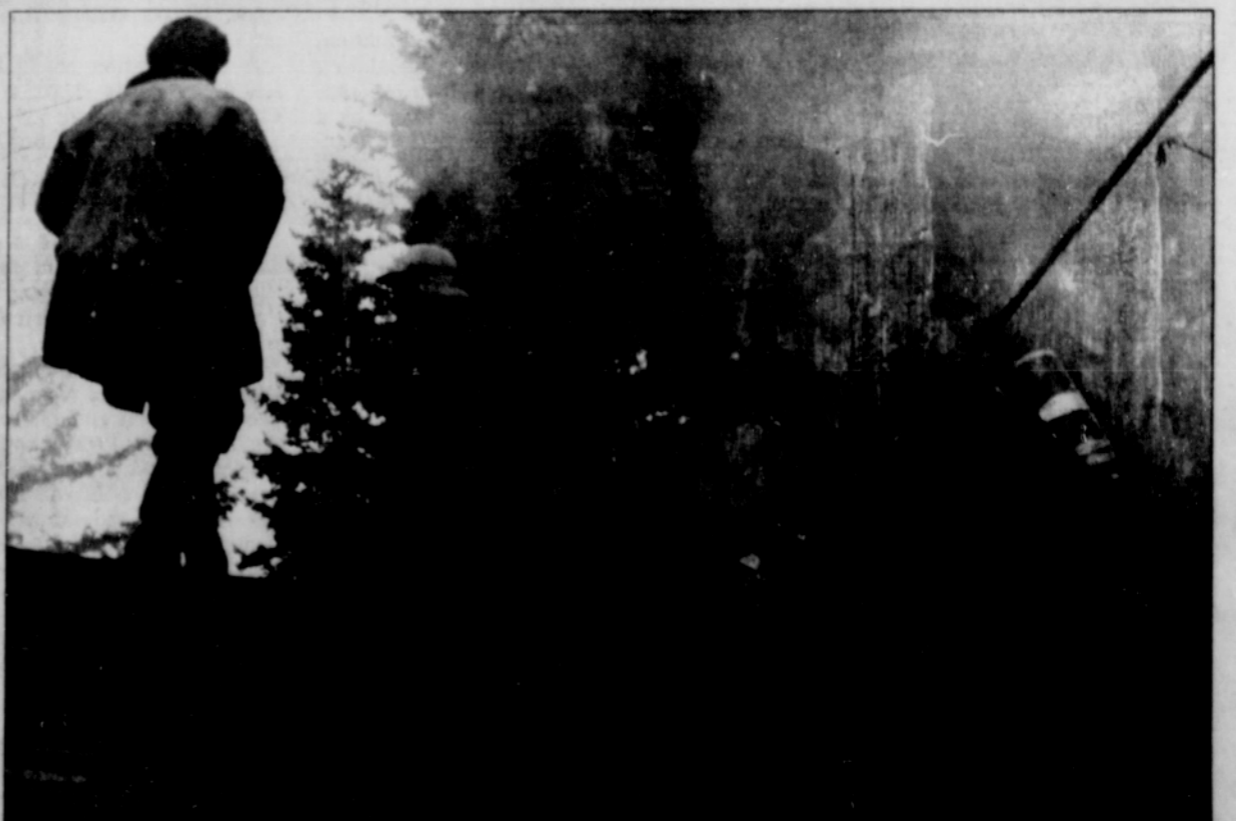
Sandy firefighter Steve Mackey vents the roof above the living room to allow smoke to escape from the attic Monday at a house fire on SE Colorado Road. Photo by Dan Dillon
