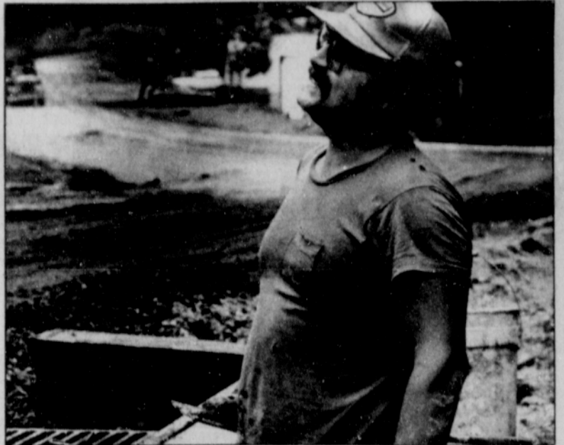
Pictured above finishing the cement on a storm sewer on Tupper Road is Rick Nelson of Portland, who works for Sharp and Associates of Beaverton, subcontractors on the job. Tupper Road, between Highway 211 and Sandy Heights Road in Sandy, will be closed beginning next Wednesday, July 7. The closure will begin at 8 a.m. and continue to 8 a.m. July 12 for road construction.
