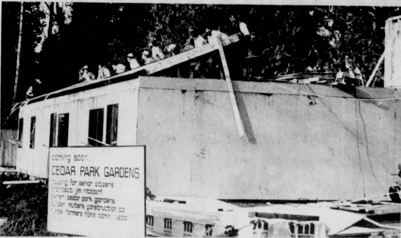
Workers put up a wall at the senior center apartment complex on McCormick Drive, adjacent to Meinig Park. The $675,000 Cedar Park Gardens will
