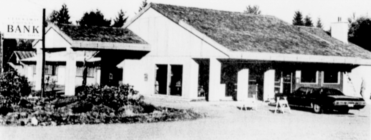
Work continues on the remodeling of the Clackamas County Bank at Welches.
