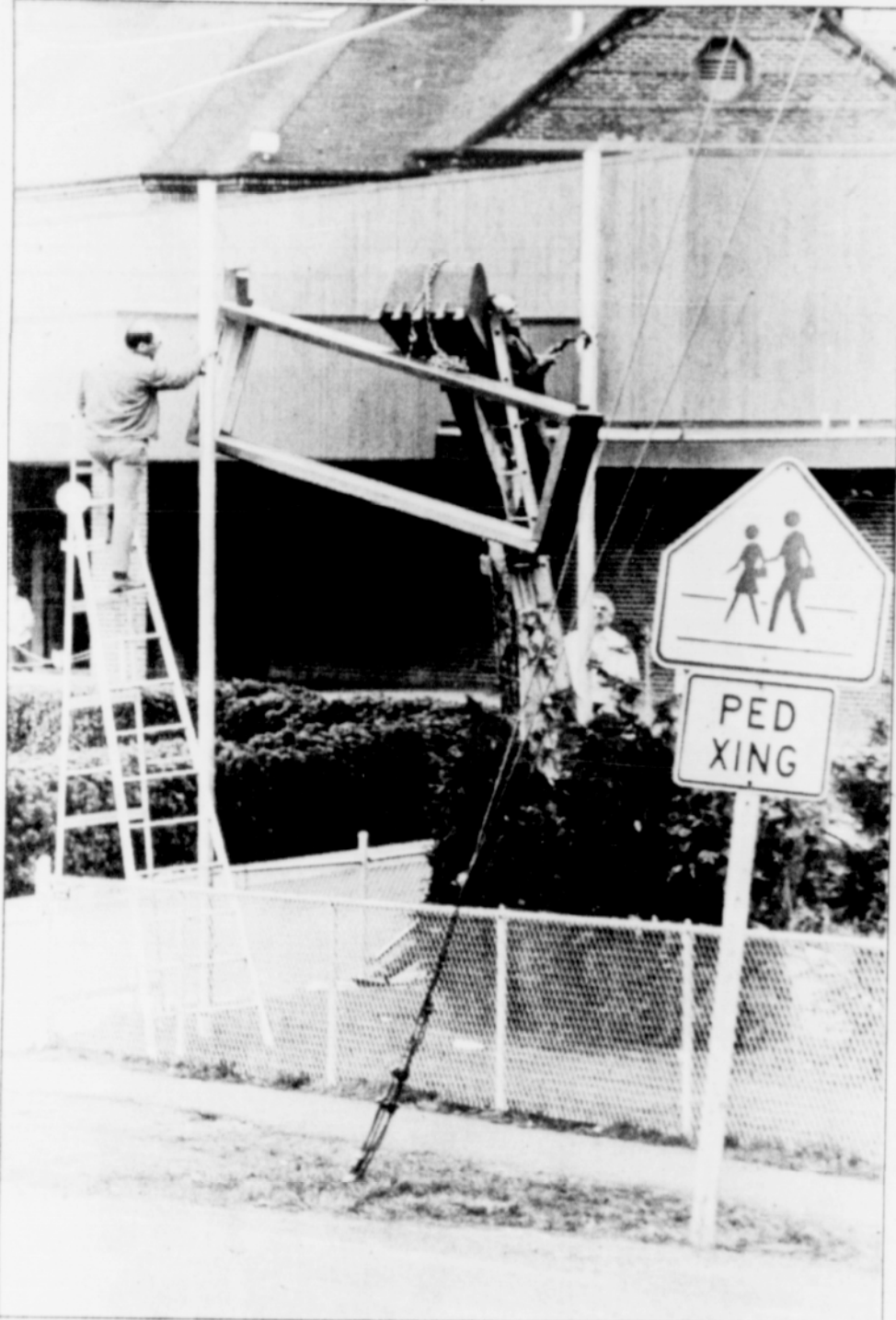
Workmen at Sandy High School re-install the school's marquee after Tuesday afternoon after it was removed for some touch-up repairs.
