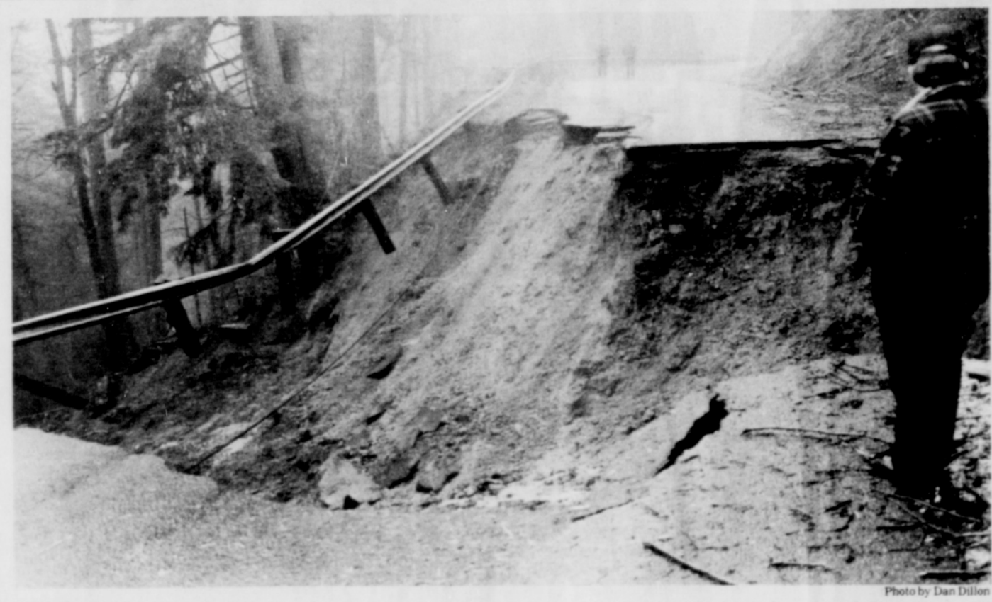
Ten Eyck Road collapsed and disrupted traffic for two and a half months.
