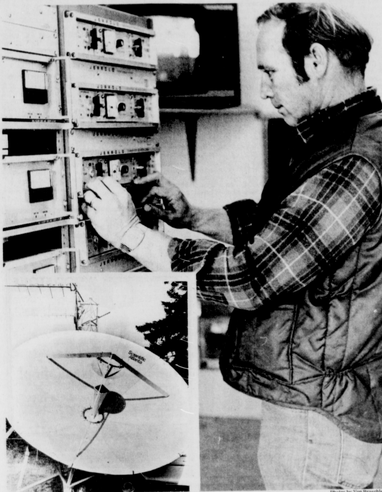
Warner Amex Cable engineer Bob Tranetzke of Sandy "fine-tunes" incoming satellite and network television signals at company's new earth station in Sandy Industrial Park. He maintains this bank of modulators and processors stored in a trailer adjacent to Warner's local antennae and giant white "dish" that picks up signals from television satellites 22,000 feet overhead. The 12-channel cable system soon will serve the Sandy area after contract delays and stalls in
