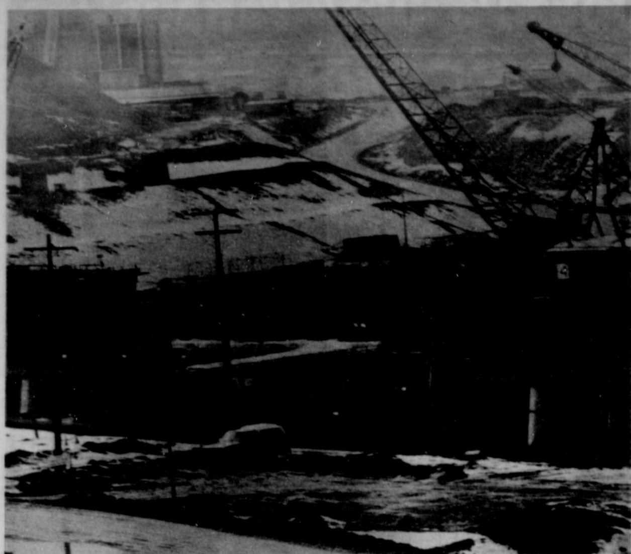
CONSTRUCTION WORK on the second powerhouse at Bonneville Dam on the Columbia River is more than two-thirds complete, according to the U.S. Army Corps of Engineers. The $575 million project, capable of meeting the electrical needs of 111,000 Northwest homes for one year, will double generating capacity at Bonneville Dam. First power from the hydro facility is due on line in May 1981 with full power by July 1982.
