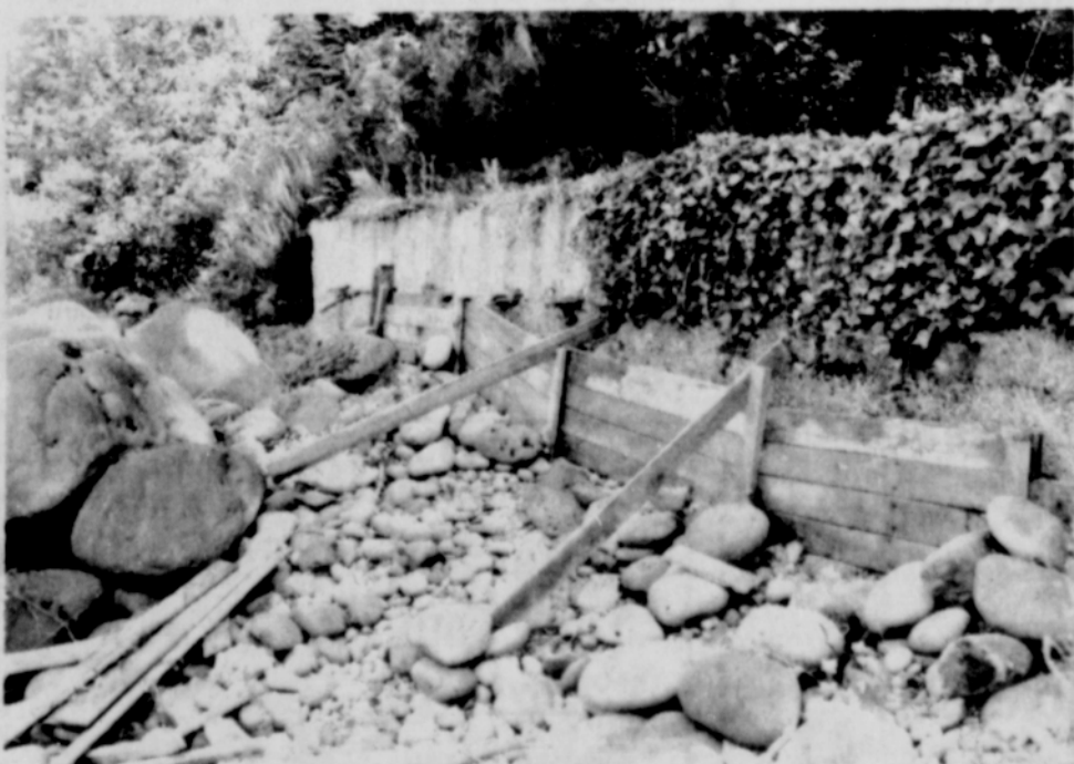
REINFORCING THE CONCRETE wall is Lee Houston's way of protecting his home against the Sandy River. Houston's property isn't specified on the
