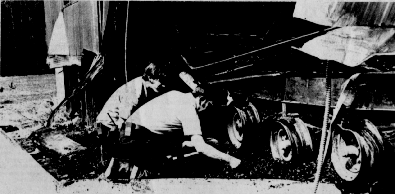
THE FIRE-GUTTED music trailer at Welches School is examined by Hoodland Fire Chief Don Armintrout (right) and Assistant Chief Lane Wintermute. Arson is suspected. The double-wide 60-foot mobile classroom serving band and choir classes was totally destroyed last Sunday night,
