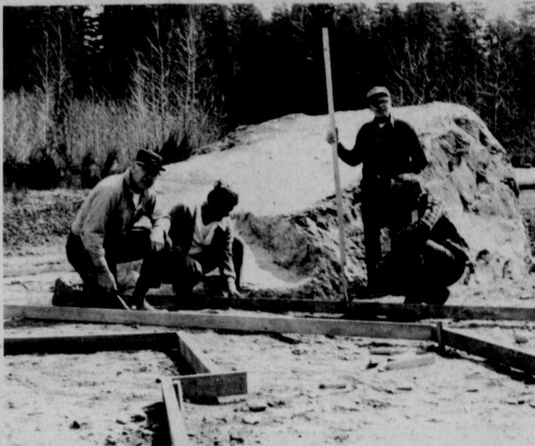
PUTT-PUTT GOLF course is being built by members the Mt. Hood Lions Club. Workers on the nine-hole course include from left Pat Kasch, Stan Lythgoe, Jack
